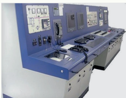
Bridge control console
