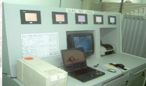
Portable Global Test Control Room – 4 units
