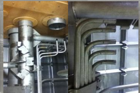
CTMS Upgrading (Capacitance to Radar)
