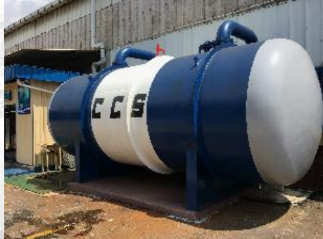
Dry-Air Tank Facility for Cryogenic Safety Valve
