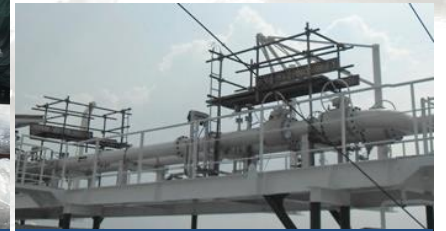
Gas Metering Skid
